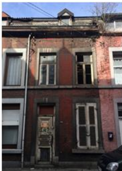
A: State of ruin Safety danger
